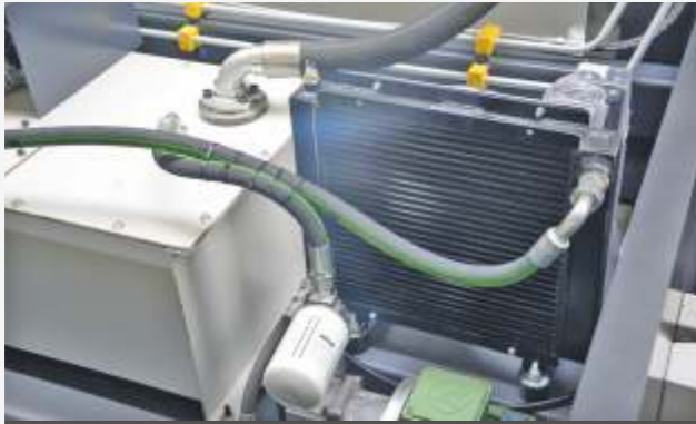
Hydraulic Oil Cooling System
